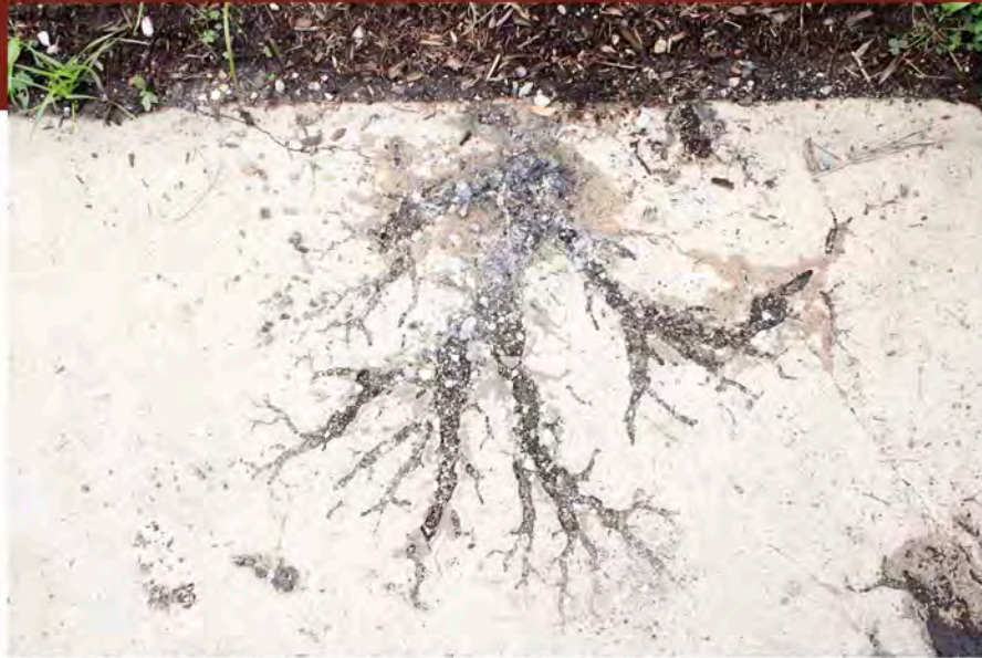
Above: Source: Mark Yingst Image taken before collecting the samples. It depicts the lightning-like pattern created in the concrete.
